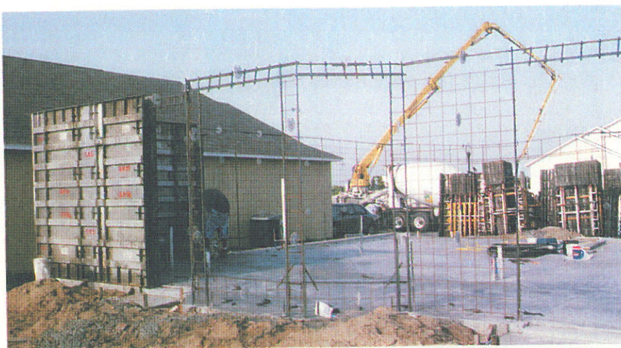
Figure 1. The author installs cast-in-place walls on the thickened edge of a slab-on-grade building platform. No. 5 rebar “up-rods” are wet-set into the slab and, once cured, wire-tied to the wall reinforcement.
