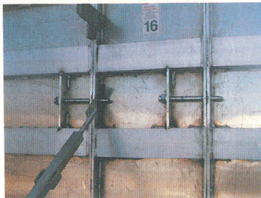
Figure 5. Attached captive pins are affixed to the face of each aluminum form on 12-inch centers. The pins pass through flat steel snap-ties before engaging the next form in line. Adjustable guide-ties enable proprietary window bucks to hang on the pins, automatically leveling the bucks in the forms.
