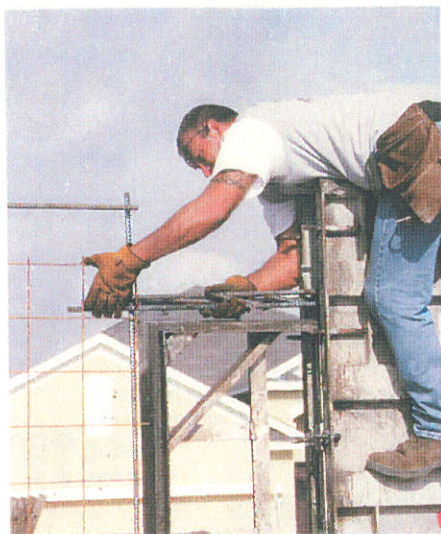
Figure 2. The typical concrete window header is 16 inches deep and is reinforced according to the particular design load.
